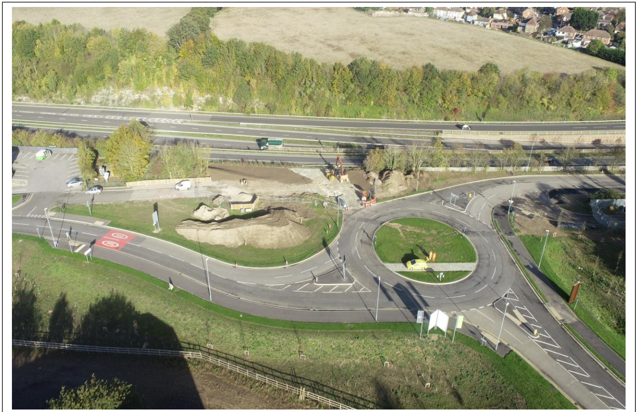
Aerial view of ongoing works on the new slip road at Chestnut Street roundabout
