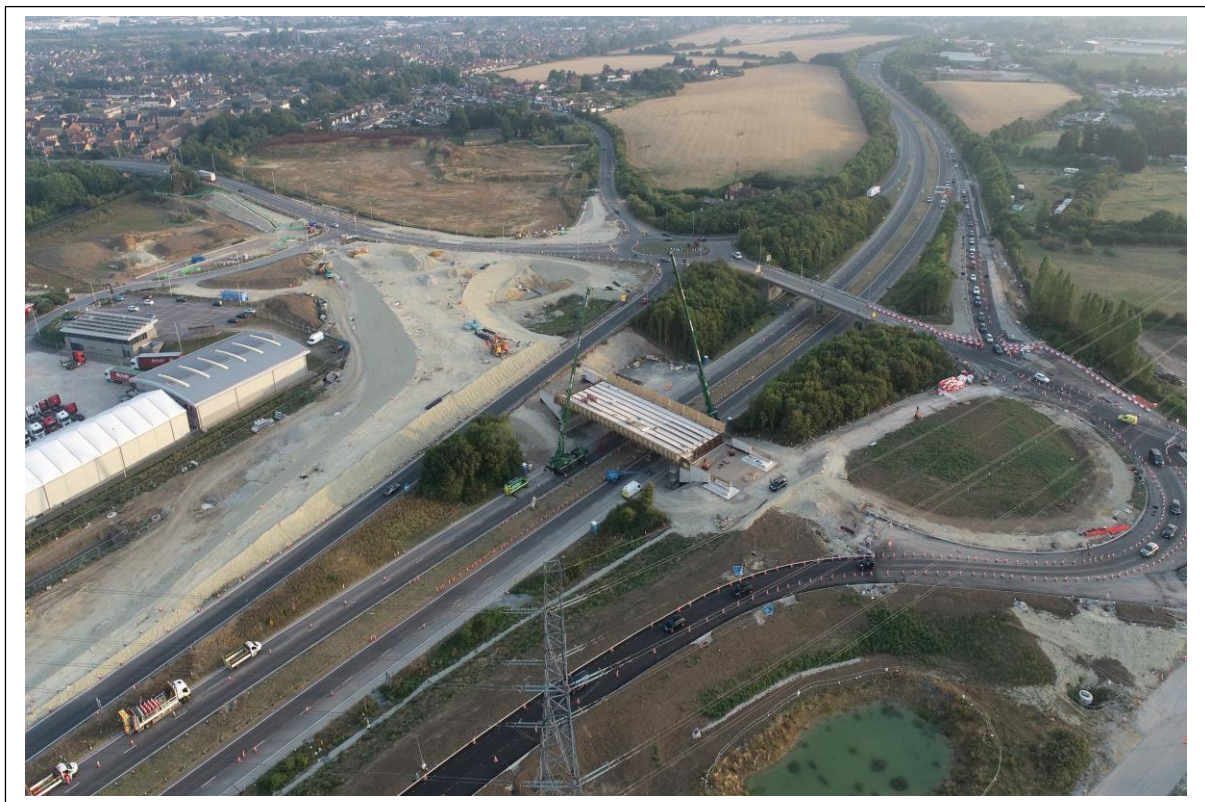
All beams and formwork for the new bridge have been successfully installed
