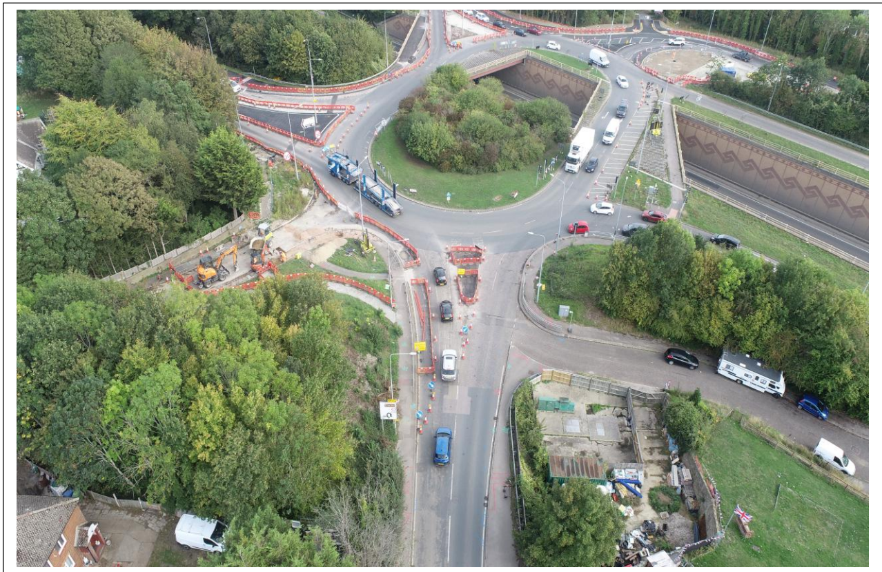
Aerial view of Key Street junction and the works progressing on Bobbing Hill
