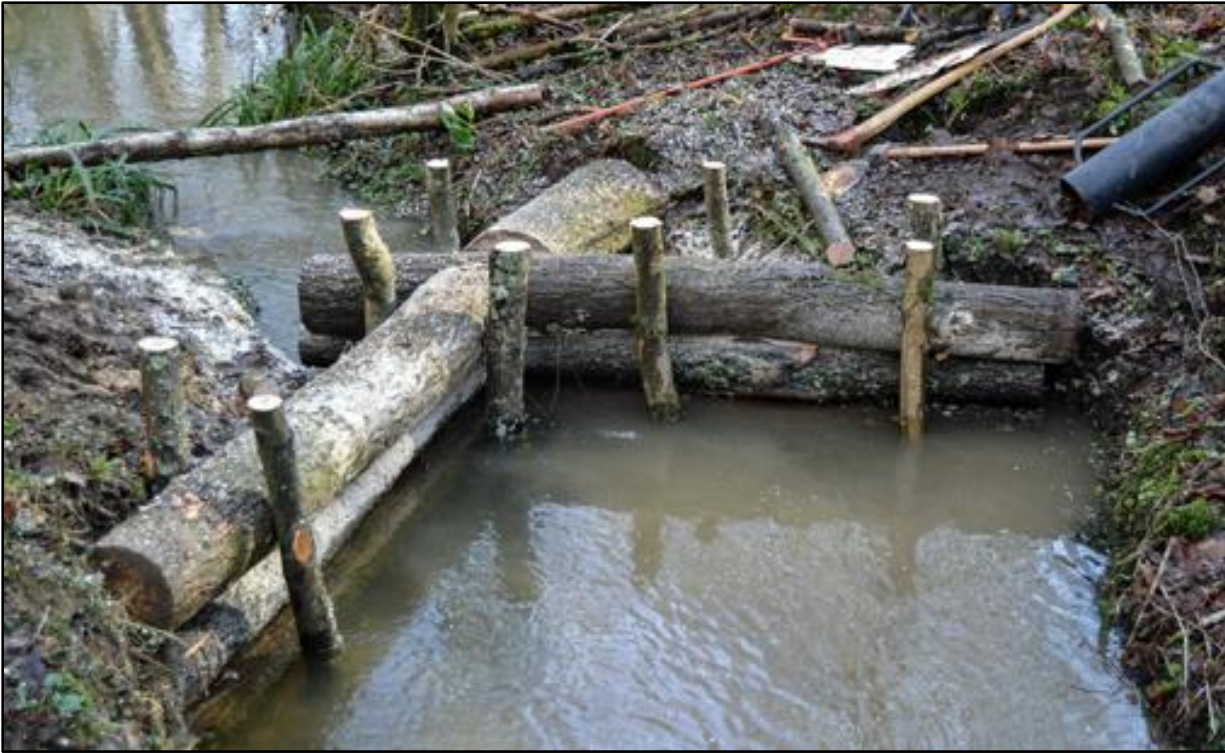
Figure 11 Leaky woody structures along the Alder Stream 7
