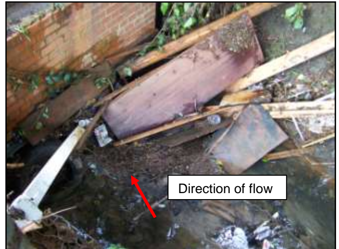
Photo.4: Rubbish & debris at trash screen (obstructed)
