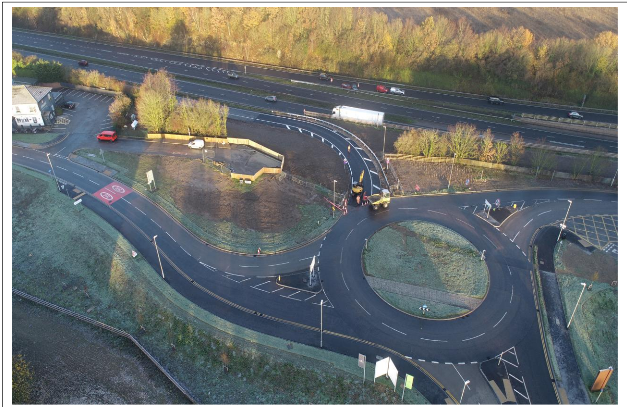
Aerial view of new Maidstone bound slip road at Chestnut Street roundabout
