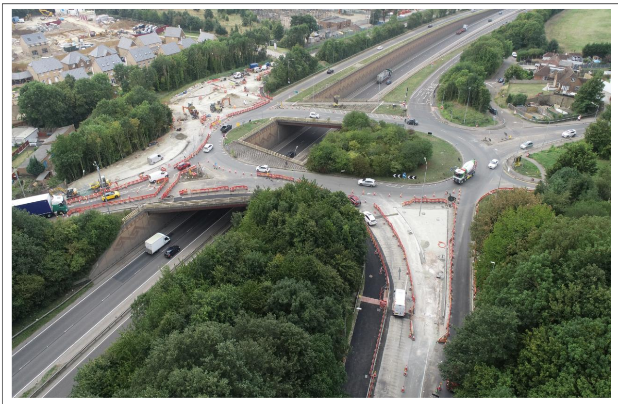
Works progressing on the realignment of Key Street / Chestnut Street from the roundabout
