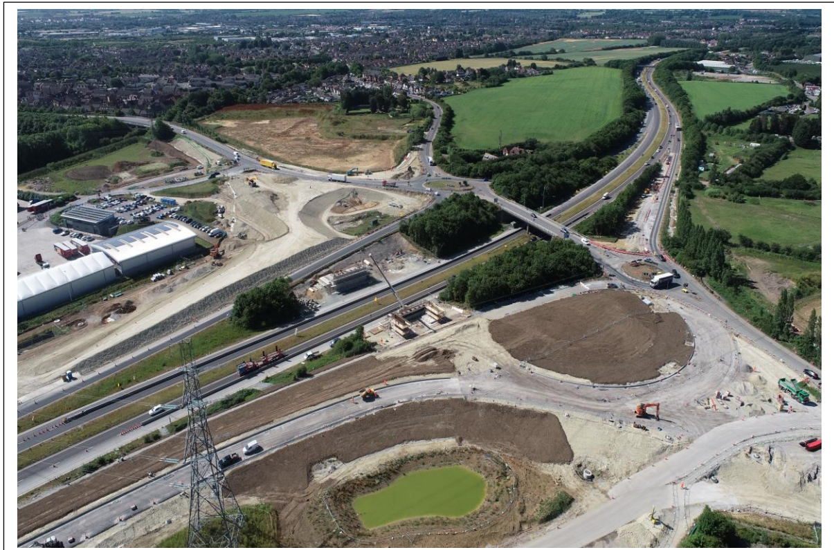
Aerial view of the new bridge walls and northbound slip roads under construction
