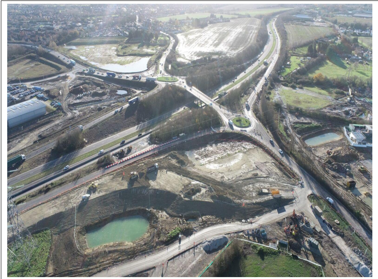
Aerial view of ongoing vegetation clearance at the site of the new Grovehurst Road Junction.
