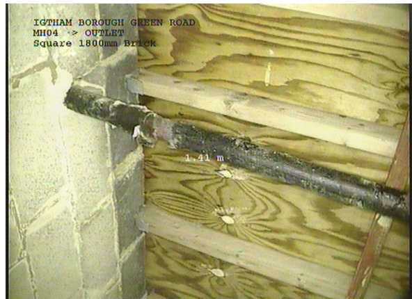
MH04X_a1c9acd0-071b-4975-8a95-800183a33cb0_20161114_102032_774.jpg, 00:01:15, 1.41m Other obstacles built into structure from 11 o'clock to 02 o'clock, 5% cross-sectional area loss
