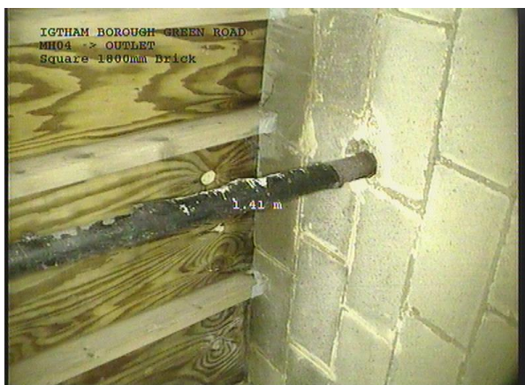
MH04X_c311e819-9a37-46d5-b2de-7bdb7525ef9f_20161114_102037_129.jpg, 00:01:15, 1.41m Other obstacles built into structure from 11 o'clock to 02 o'clock, 5% cross-sectional area loss
