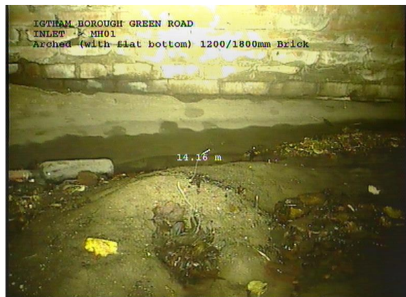
INLETX_dbe71eaf-07e2-4776-8e86-9d4848f313a7_20161114_095611_904.jpg, 00:03:15, 14.16m Settled deposits, coarse, 20% cross-sectional area loss
