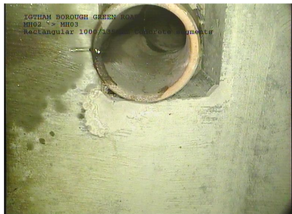
MH02X_304ea65e-93e2-4865-a823-9201b6f5fa9b_20161114_100511_780.jpg, 00:01:27, 8.56m Connection intruding at 10 o'clock, diameter: 150mm, intrusion: 5%
