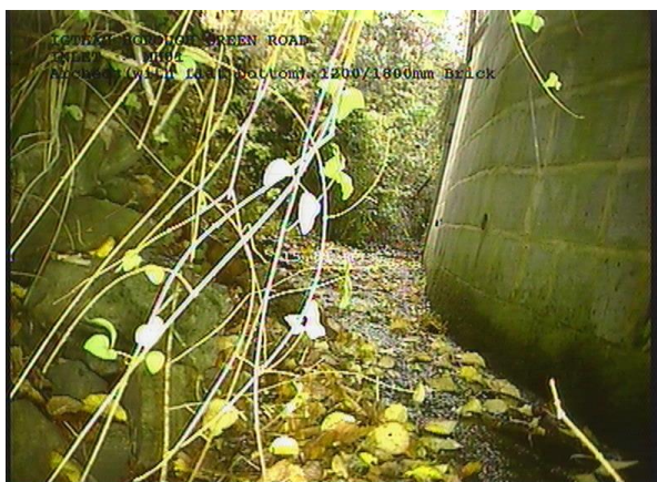
INLETX_ccb3dfaa-5be9-4866-a748-c41bfcc72aa7_20161114_095723_352.jpg, 00:04:00, 15.81m Finish node type, other special chamber, reference number: INLET
