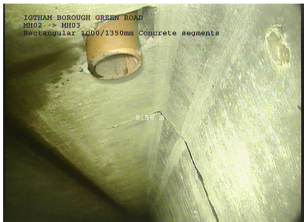
MH02X_d704efd6-ee46-41d1-b0aa-a951260c3a5e_20161114_100459_713.jpg, 00:01:27, 8.56m Connection intruding at 10 o'clock, diameter: 150mm, intrusion: 5%
