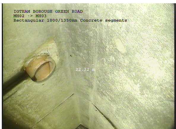
MH02X_9c2c371f-3d1e-429e-88b2-01d9fe6ff60d_20161114_100627_951.jpg, 00:02:45, 22.32m Connection intruding at 10 o'clock, diameter: 150mm, intrusion: 5%
