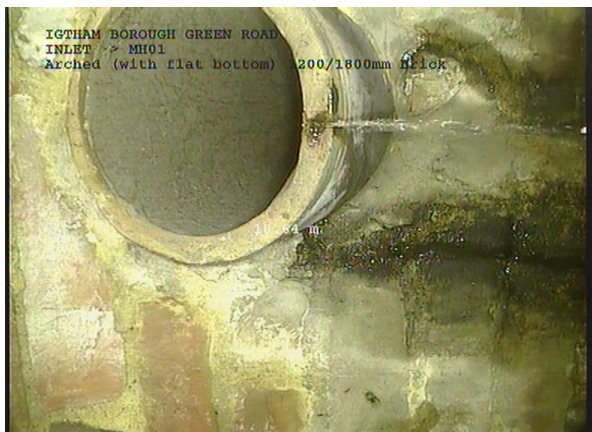
INLETX_72077c10-7042-4751-82e1-27c15a969910_20161114_095435_547.jpg, 00:01:39, 9.77m Connection intruding at 01 o'clock, diameter: 150mm, intrusion: 5%
