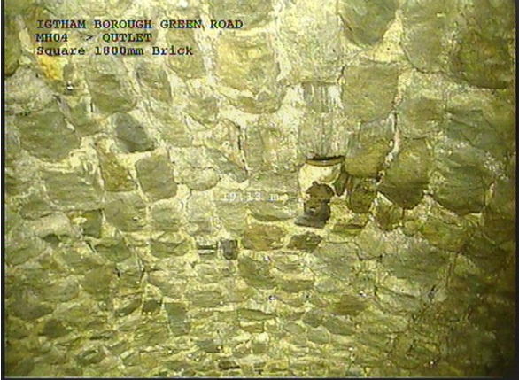
MH04X_b9e8755f-3052-4963-a466-8bca00524ba2_20161114_102612_724.jpg, 00:05:18, 19.13m Connection other than junction at 03 o'clock, diameter: 100mm
