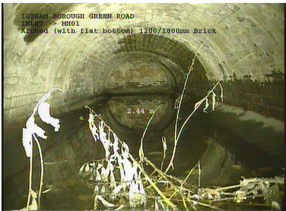
INLETX_367b83e1-5855-489c-9d90-cde203426b86_20161114_095304_525.jpg, 00:00:46, 2.44m Settled deposits, other, 10% cross-sectional area loss
