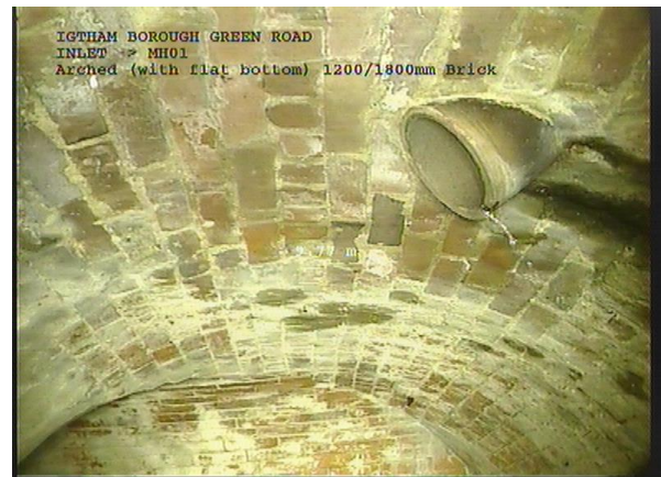
INLETX_dc62b6e1-1a08-4282-a23e-f4690d841a61_20161114_095412_419.jpg, 00:01:39, 9.77m Connection intruding at 01 o'clock, diameter: 150mm, intrusion: 5%
