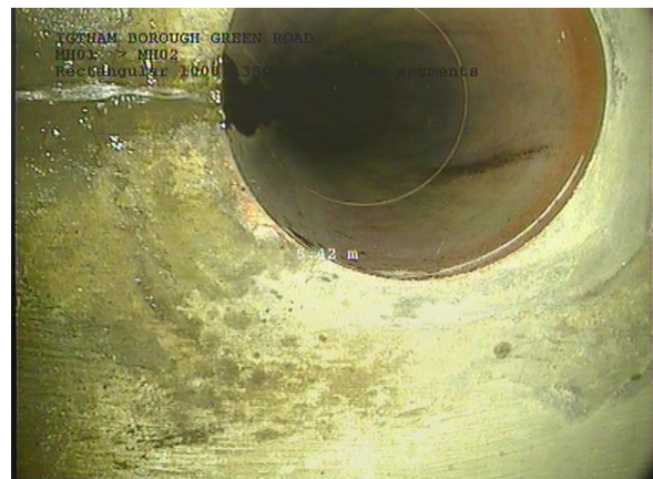
MH01X_1f7062c0-f8a2-4e4a-8660-cb3a70676c46_20161114_094257_413.jpg, 00:01:07, 4.76m Junction at 09 o'clock, diameter: 300mm
