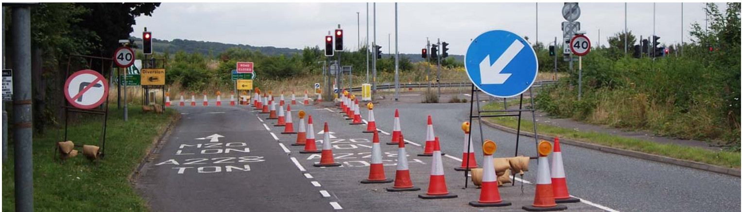
Castle Way junction with A228 Leybourne & West Malling Bypass with temporary ban of right turn movement
