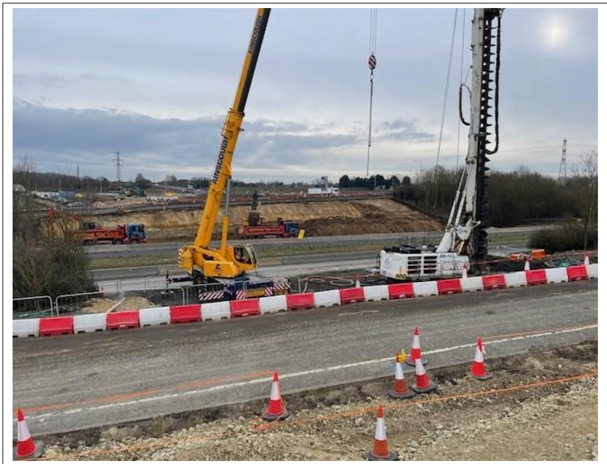
Piling works ongoing at the site of the new A249 Grovehurst Road junction.
