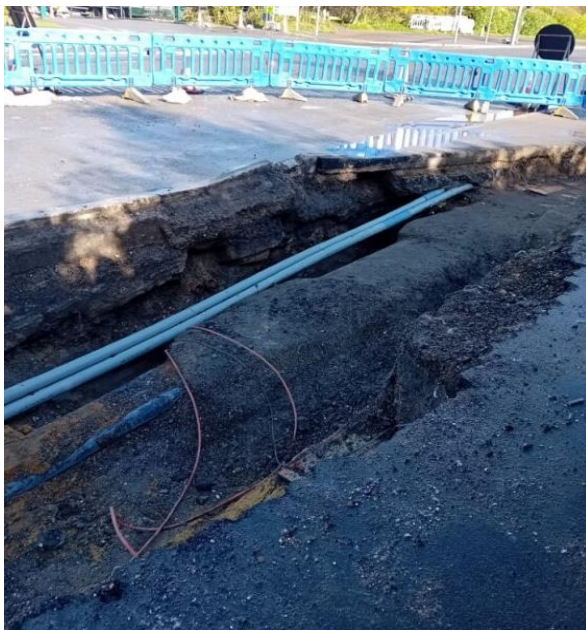
Existing BT cable exposed and chased.
