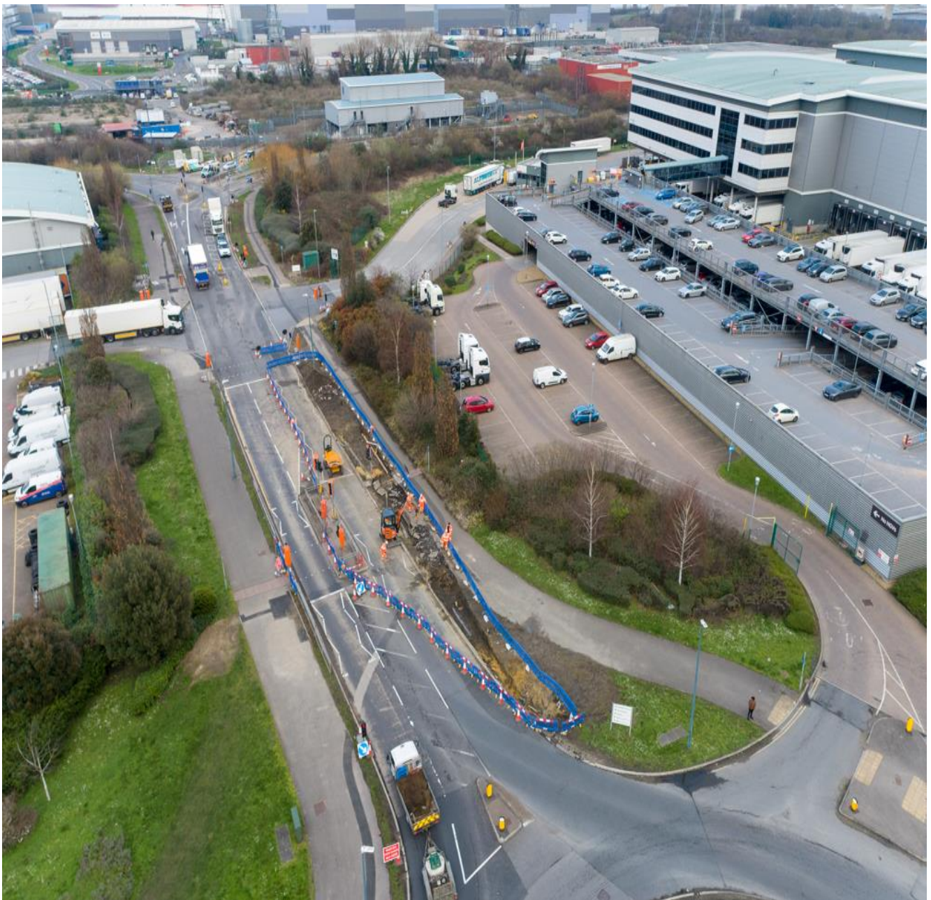
Aerial shot of Rennie Drive construction works looking north towards The Bridge Estate.
