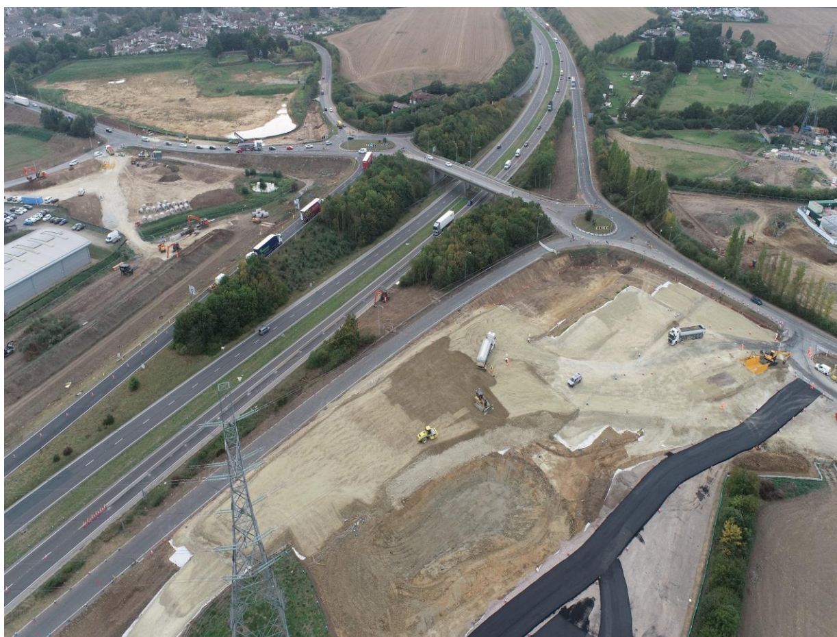
(Drone image of the current A249 Grovehurst Road Junction, showing ongoing vegetation clearance and works for setting up a permanent construction site compound)
