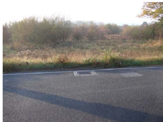
Depression adjacent to Shalmsford Street
